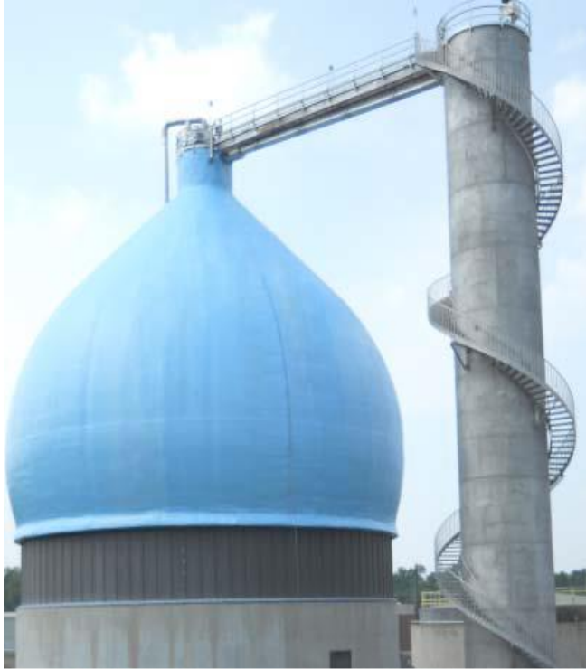
Figure 5. DTMA's egg-shaped digester. Source: DTMA.
