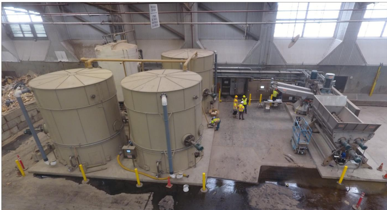
Figure 2. In the Doda food scrap processing facility at the Puente Hills MRF, food scraps enter the Doda equipment (right); after preprocessing, the slurry is stored in storage tanks (left) until it is pumped to the digesters. Source: LACSD.
