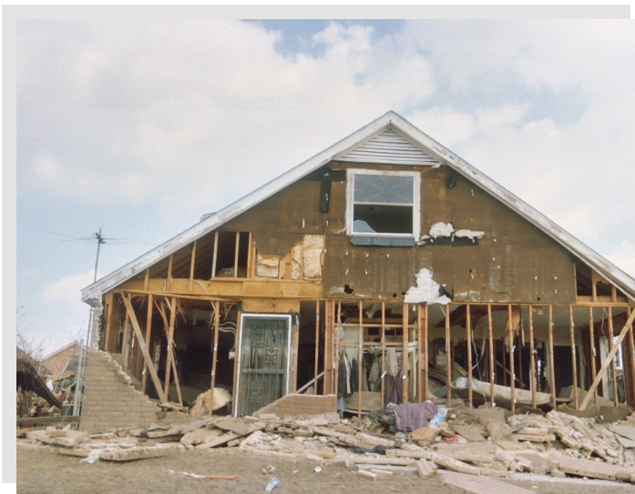
New Orleans home after Hurricane Katrina. Photo by Lawyers Committee for Civil Rights Under Law.
