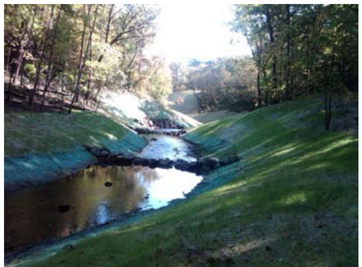
Scott WMO, working with the City of Savage and Scott SWCD, received $130,000 from the Clean Water Fund to install this BMP to stabilize the Utica Ravine, and help restore the Credit River.
