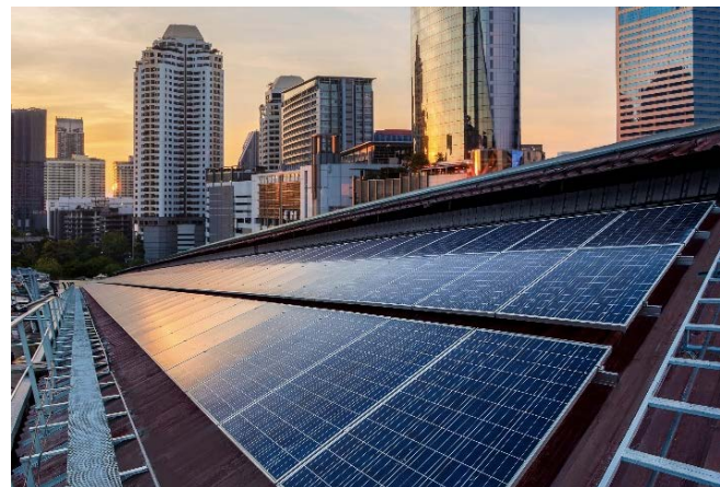
Rooftop Solar Installations
