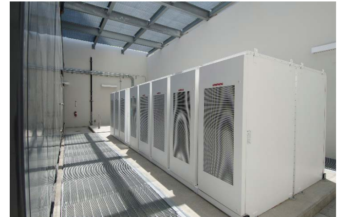
Battery Energy Storage Systems
