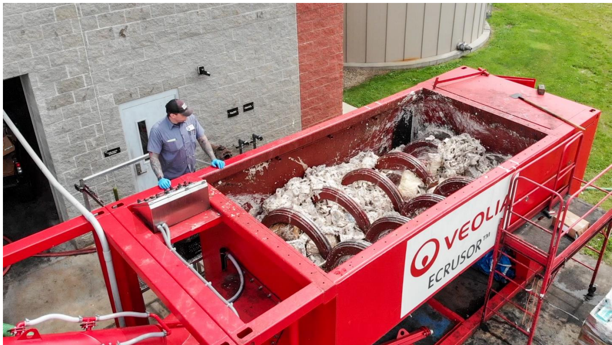
Veolia ECRUSOR™ preprocessing equipment in the Food Waste to Energy Recovery Facility. Source: HMA.
